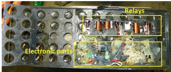
Figure 4 – The verification switch and abnormal electronic devices hidden under the epoxy resin [15]
